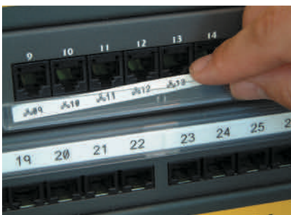
Punch Block & Patch Panel Labels
