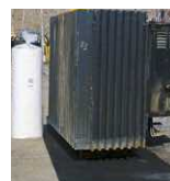
Ideal underneath leaking transformers.
